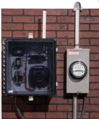
Wall mount with cooling Fan
